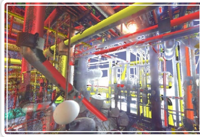
EdgeWise was able to accurately extract and model nearly 70% of the scanned pipes.
